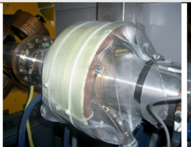
WALL CURRENT & DCCT MONITOR
