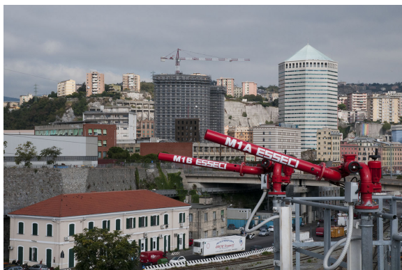
Foam system - Port of Genoa - Italy
