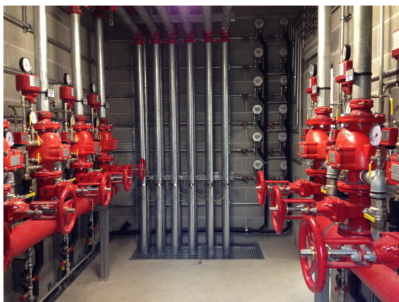
Dry sprinkler system - Business District "Piero della Francesca" - Turin - Italy
