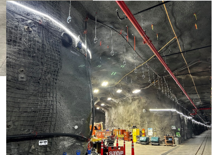
Plumbing, Fire Suppression and Smoke Detection
