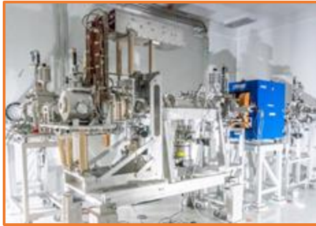
SPES ISOL bunker (already installed!)
