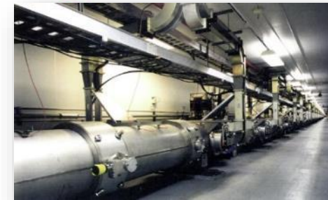
Cryomodules in the accelerator tunnel
