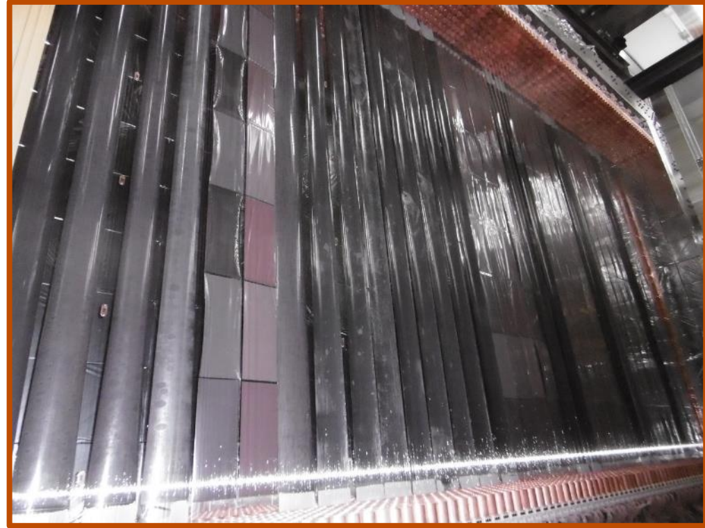
Picture of installed source foils
