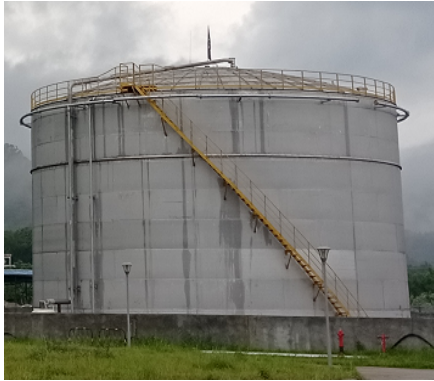
5000 m 3 LAB tank
