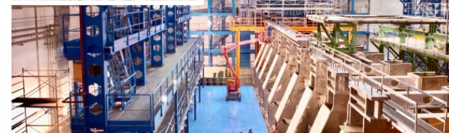
LAr endcap presampler installation (2005)
