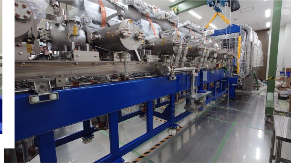
Picture 2-26: Cold mass during lifting test in JR building
