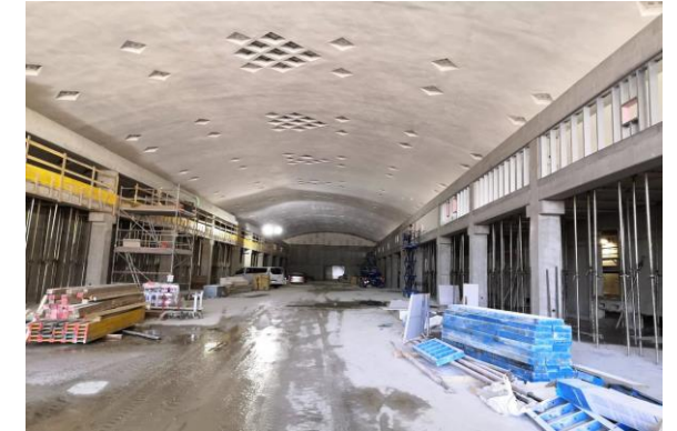
Each of the 6 “botti” (barrels) is ~5000m 2 of usable IT space
