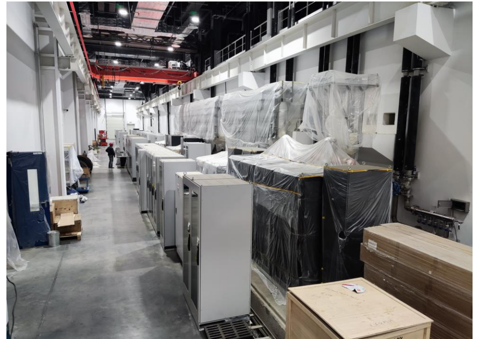
Electrical and RF power source gallery
