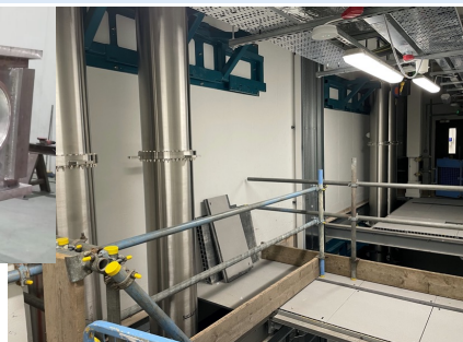
Riser pipework – Ground floor corridor
