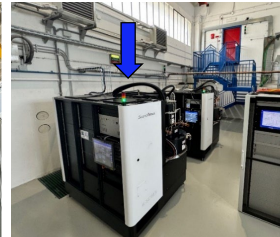
Installation at TEX
