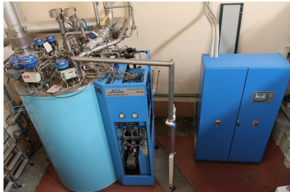
LINDE He refrigerator/liquefier
