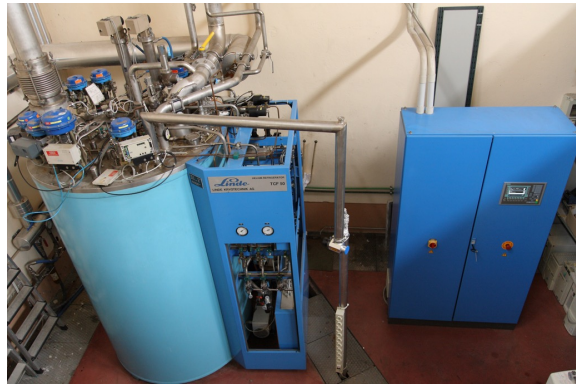
LINDE He refrigerator/liquefier
