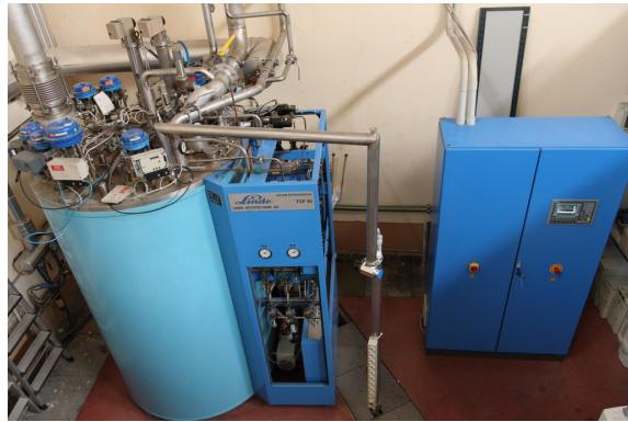
LINDE He refrigerator/liquefier
