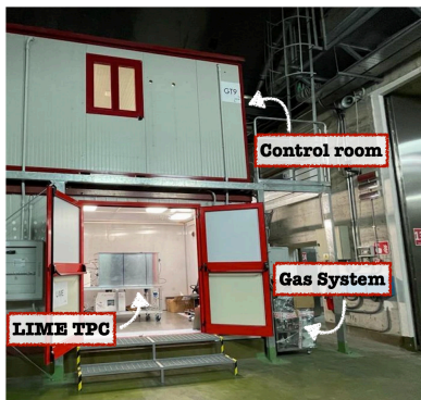
Underground installation with full auxiliary systems
