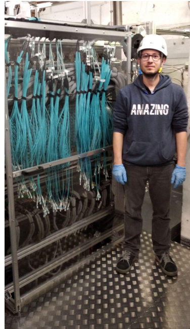
LHCb VeLo Recabling & Recommissioning (Feb.)
