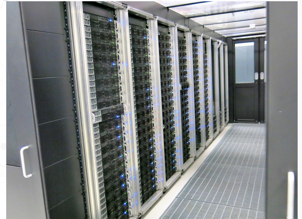
SERVER ROOM ReCaS-Bari ( https://magnanimo.it/progetti/terziario-ed-industria/infn---recas-bari.html )
