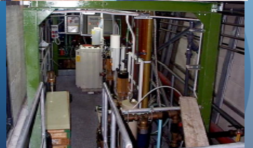
Water purification system
