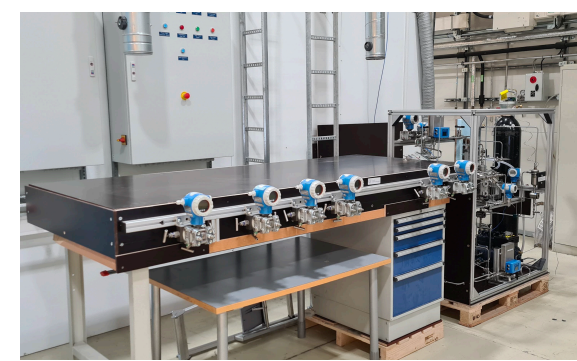
Cold detectors: Kr / sKr facility
