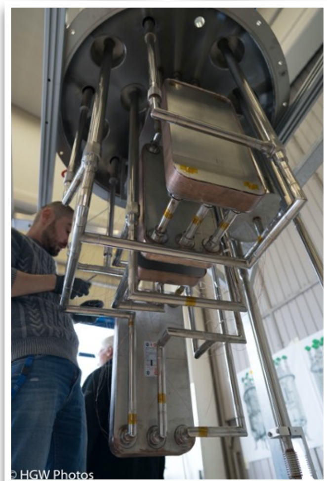
In-house fabrication of the gas handling system
