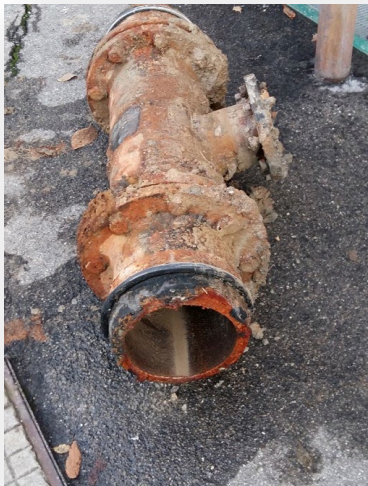
The broken pipe
