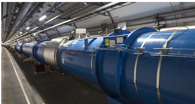
LHC dipoles (8 T) in the tunnel
