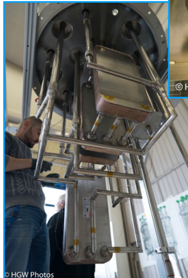
In-house fabrication of the gas handling system
