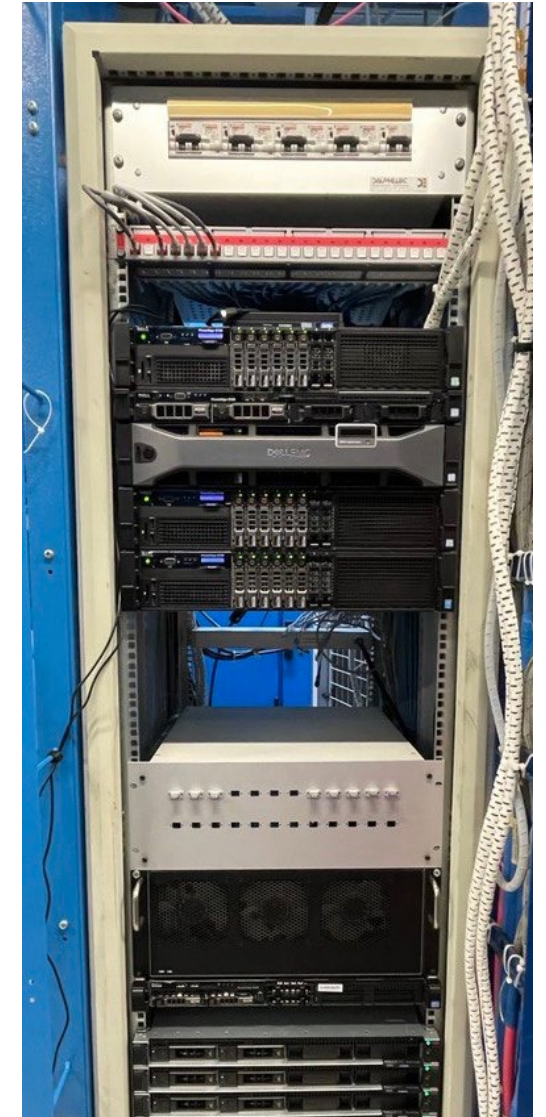
Level-1 Data Scouting rack
