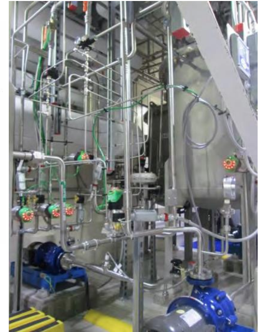
LS purification plant
