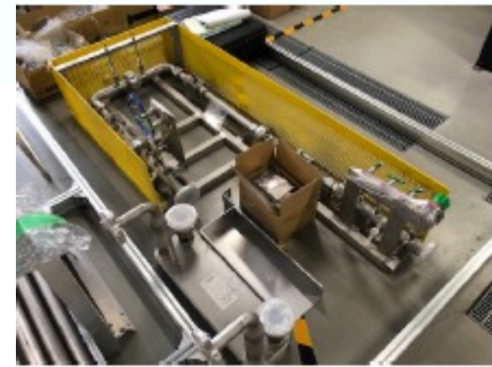
New target cooling system
