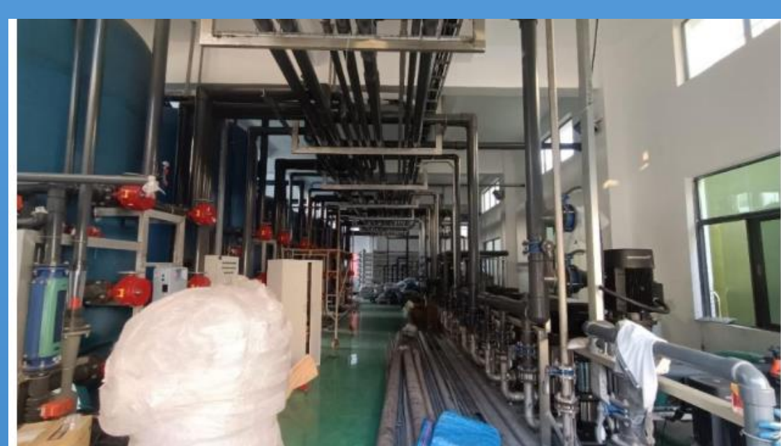
Water system (ground)
