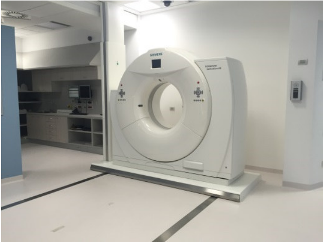
CT on rail in one Gantry room
