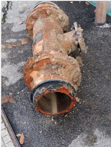
The broken pipe
