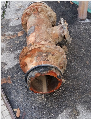
The broken pipe
