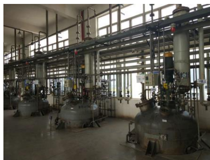
Special pipeline for MMA
