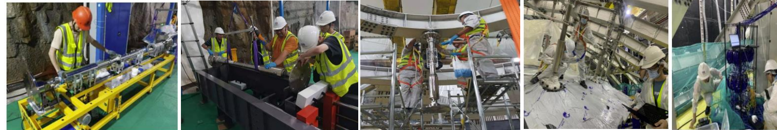
Connection process: sensor installation and test → connected with SS → with acrylic → pre-loading → unloading the fixtures, transfer acrylic weight to the bars → monitoring load
