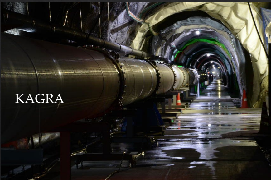
Tunnels and vacuum pipes
