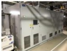
New Horn PS/ trans/strip-lines for 320kA & 1Hz
