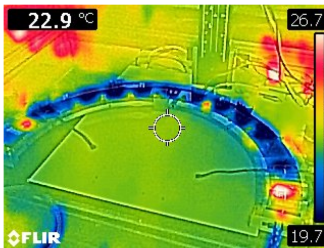
Figure 111: Thermal image of the Genova half-ring with the two ITkPixV1 modules powered by the V6 bus tape.
