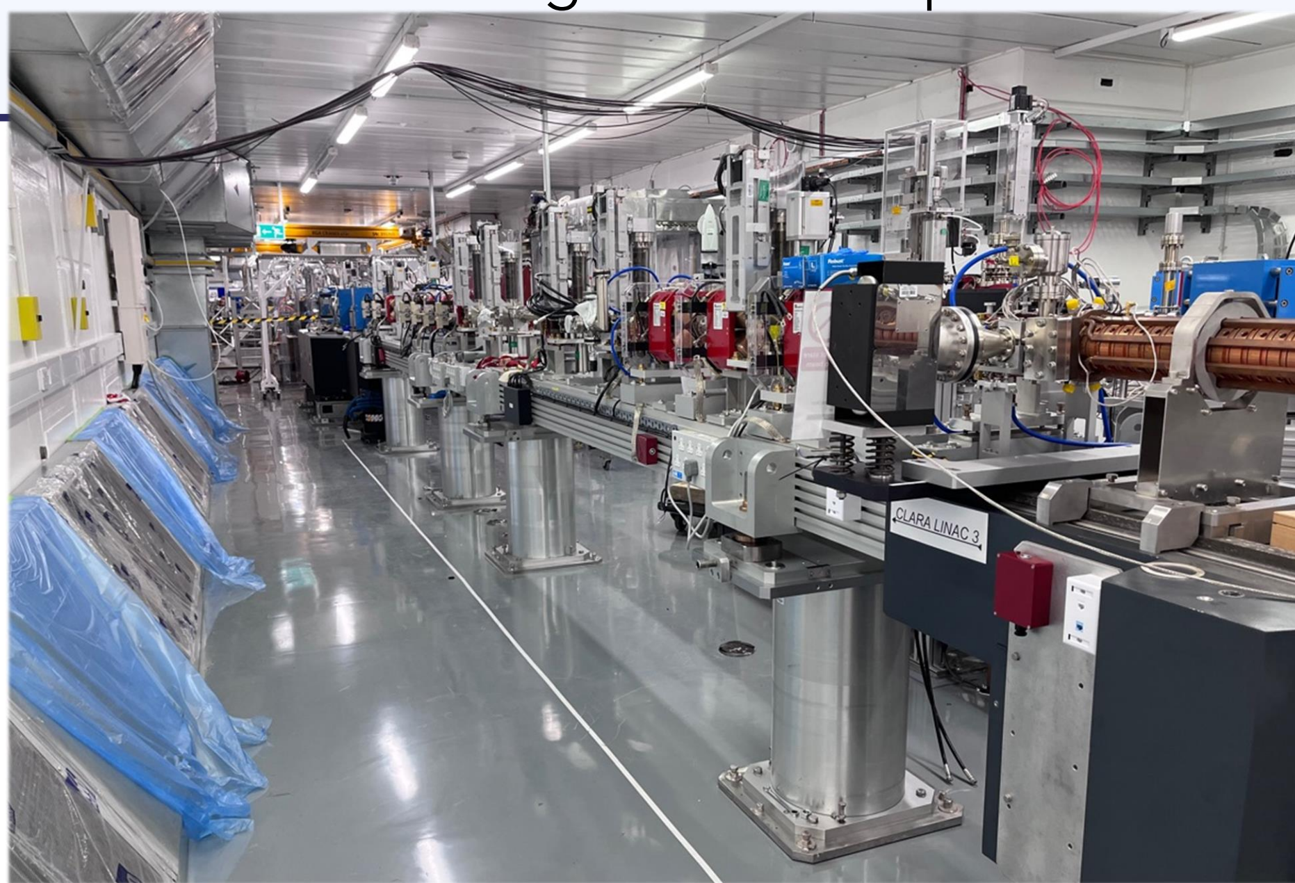
Figure 4: Completed installation of CLARA linac modules in the main accelerator hall.
