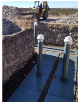
30 m 2 buried scintillators
