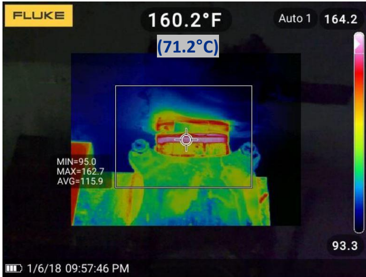
IR camera image of the bottom of the penetration
