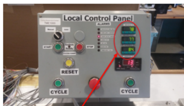
Cooling water temperature panel
