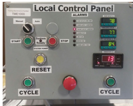
Figure 21: Cooling water temperature control panel.
