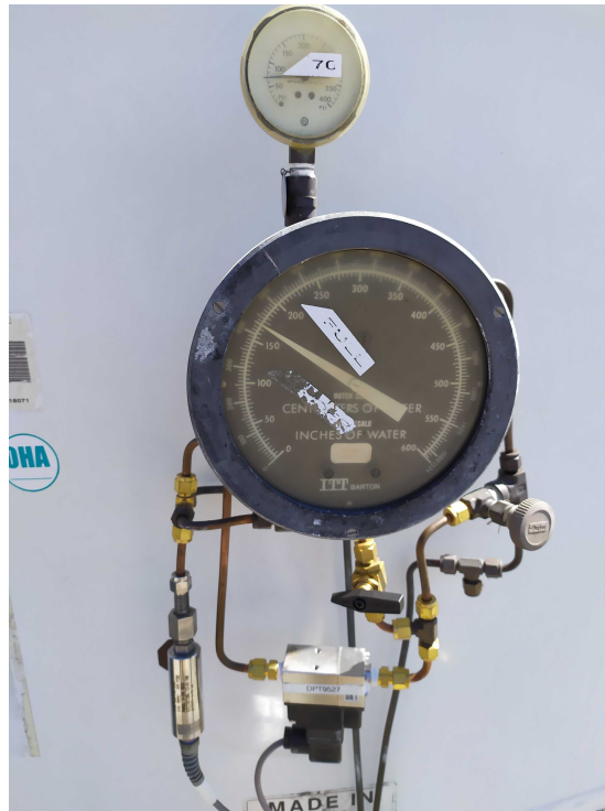
Figure 16. Pressure sensors of Tank 15. The small dial gauge measures the absolute top pressure; the big dial gauge measures the differential pressure; the left transducer reads the absolute pressure; the right transducer reads the differential pressure.
