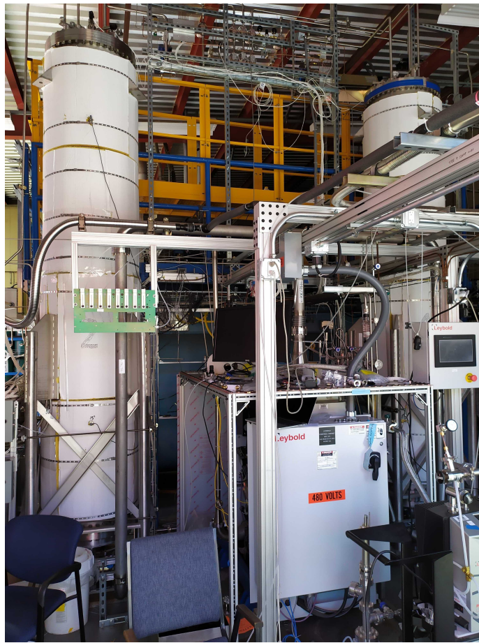
Figure 8. Picture from the removal system, the two white charcoal columns (left and right) and one of the circulating pumps (middle) are visible.
