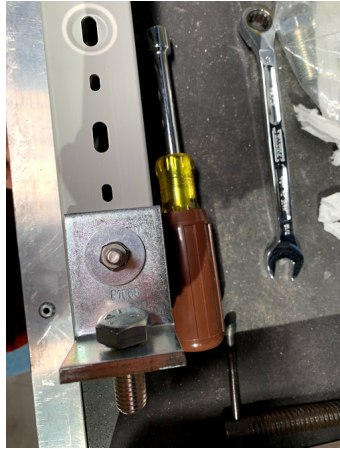
(a) Preparation of the cable trays, before the assembly on the mezzanine floor.
