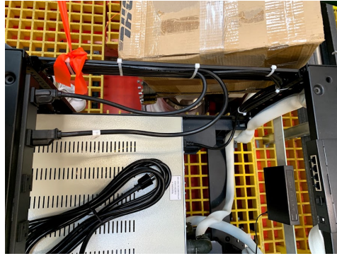
(b) Cables secured on the left side of the frame.
