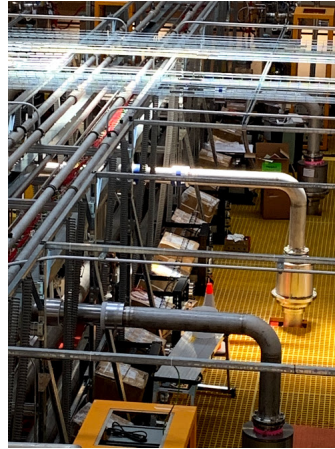
(b) Cable trays installed along the whole length of the detector.
