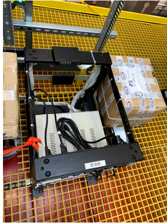
(a) Top view of a cabled mini-rack (Ethernet cable missing).
