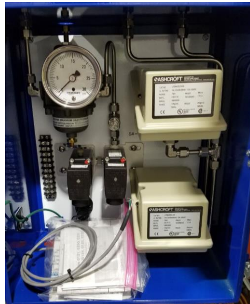
BTM Control Box (as built)
