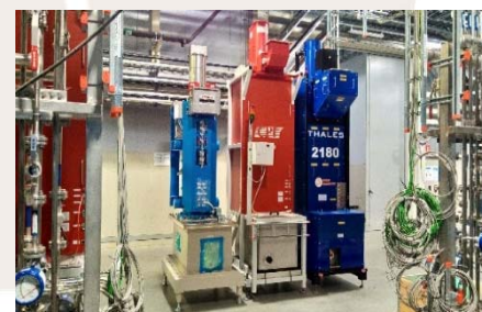
Klystrons used at ESS
