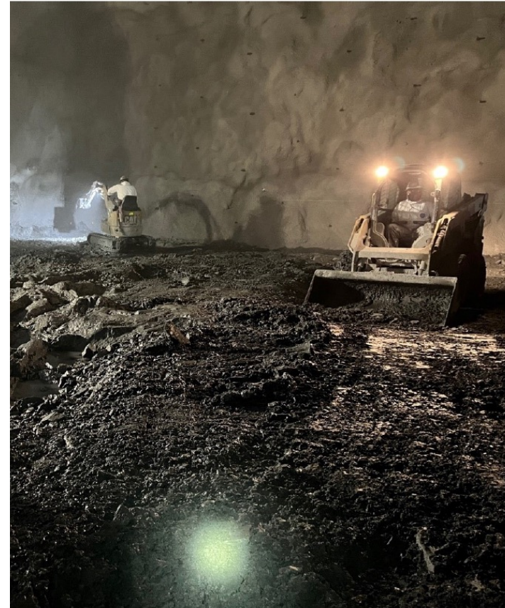
Blow piping central utility cavern
