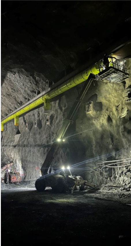
North Cavern – adjusting ventilation
