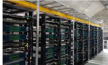
underground electronics room
