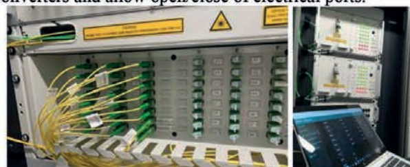
Figure 3: Left- the optical patch panel of the IDMAR RCB with 22 fibers to CTF-02 connected together with the 2 control fibers (positions 23 and 24); Right- the RCB synoptic panel to control the CTF-02 and (when available) CTF-03. The system is fully redundant.
