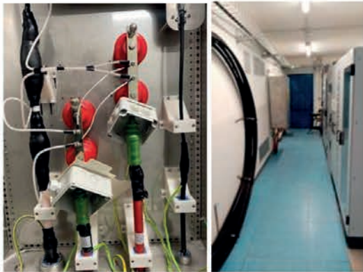
Figure 4: Left-The inner part of the SBJ, where the MEOC is split into 2 conductors and separated by the fiber bundle. Right – the IDCAR DCFO room
