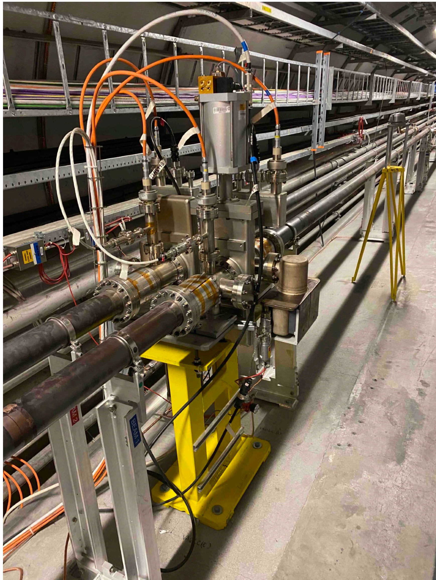
Sector valve to isolate the region
