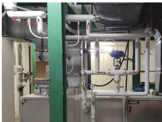
New Cooling Water Distribution System
