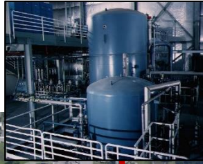
Cryogenic Refrigeration Plant
