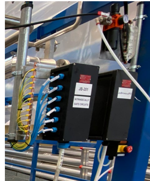
Junction boxes on skids
