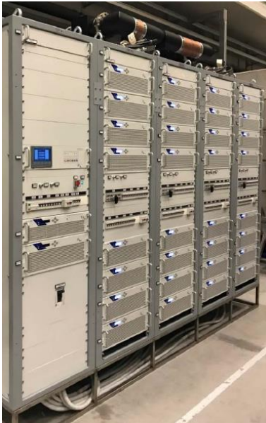
INFN solid state amplifier (125 kW cw, 352 MHz), 5 machines built for MUNES project in the national industry (2017).
